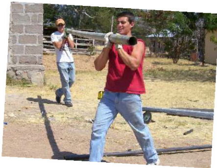
Robert and Anthony working on soccer goals... building the new soccer field was a huge blessing to the school
